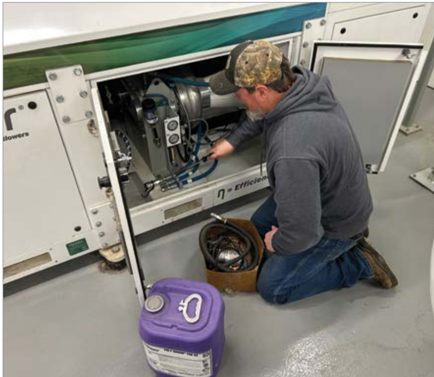
Plant Operator Brett Benefield performs an annual oil and filter change at Plant No. 3.
