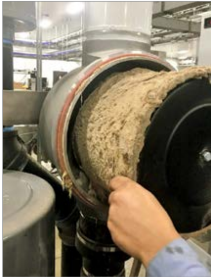
Filter neglect at a Chicago food packaging facility led to significant replacement costs and hours of downtime.
