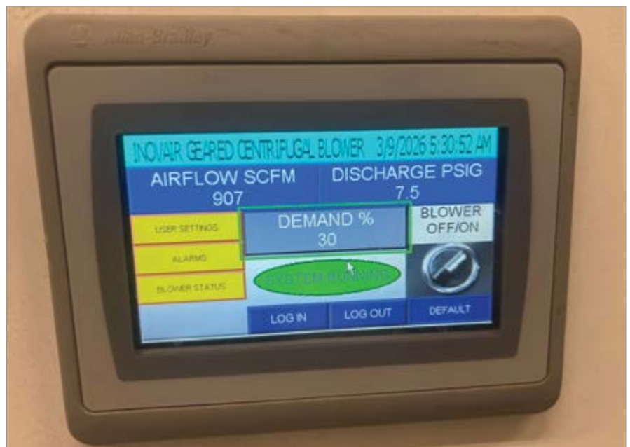
An MCP shows the status of a blower at Plant No. 3.
