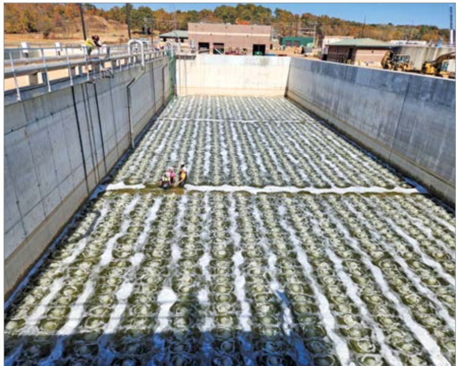
A fine bubble aeration basin at startup.
