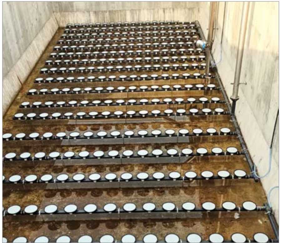
This aeration basin has coated membranes for a longer lifespan and reduced maintenance.
