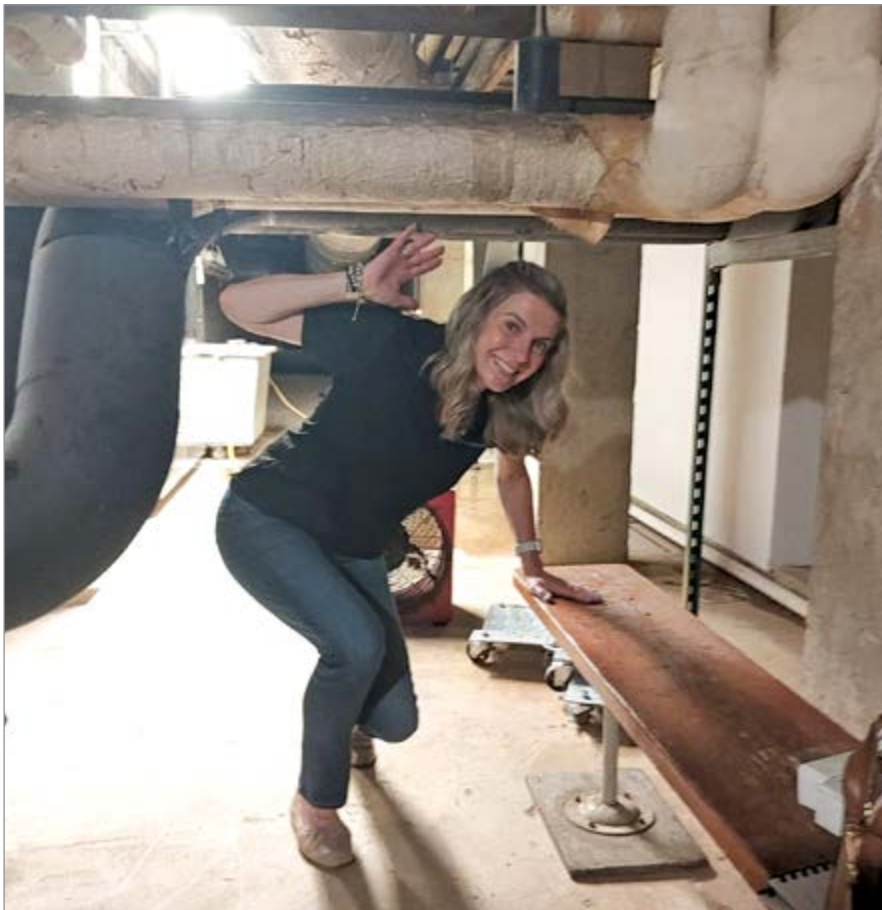
Elizabeth Fleming demonstrated the narrow passage for the duplex vacuum pump system’s installation.
