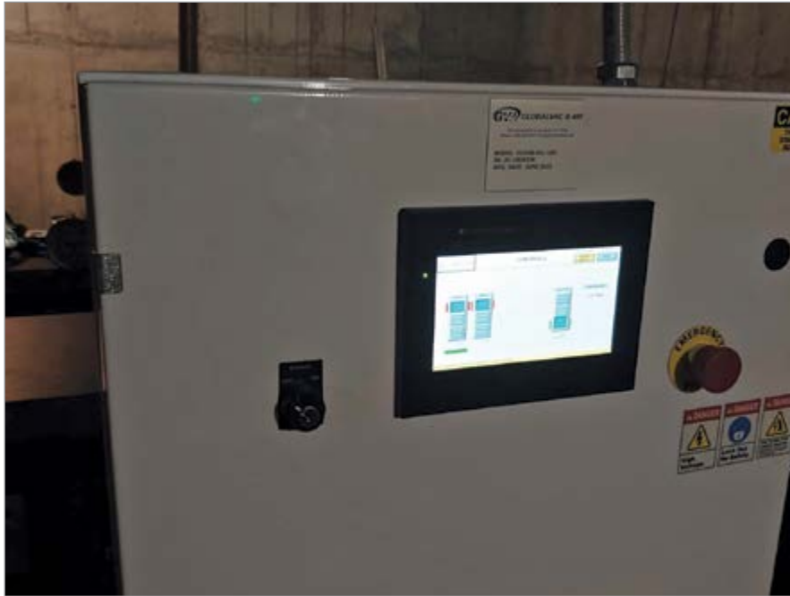
The duplex vacuum system's control panel offers a touchscreen interface.
