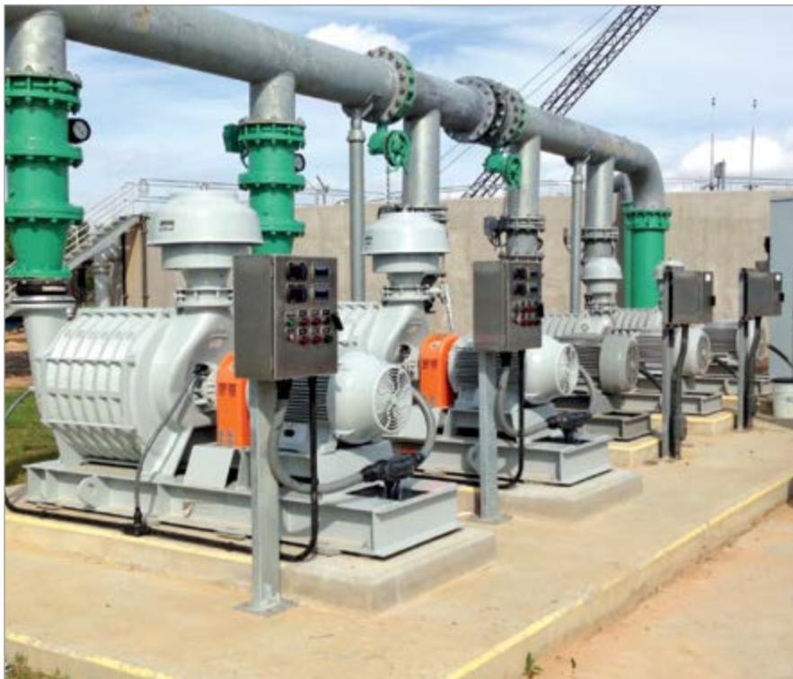
An aeration blower system used by a food processor.
