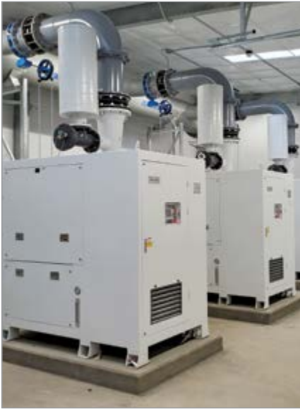
These turbo aeration blowers were installed in a food processing plant in Washington in 2020.
