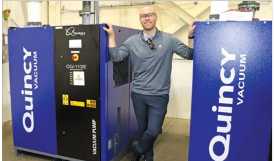
Account Representative Bryan Dominick with the two newly installed VSD vacuum pumps.
