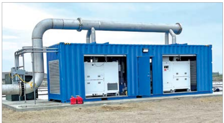
Turbo aeration blowers at a major sugar refinery.
