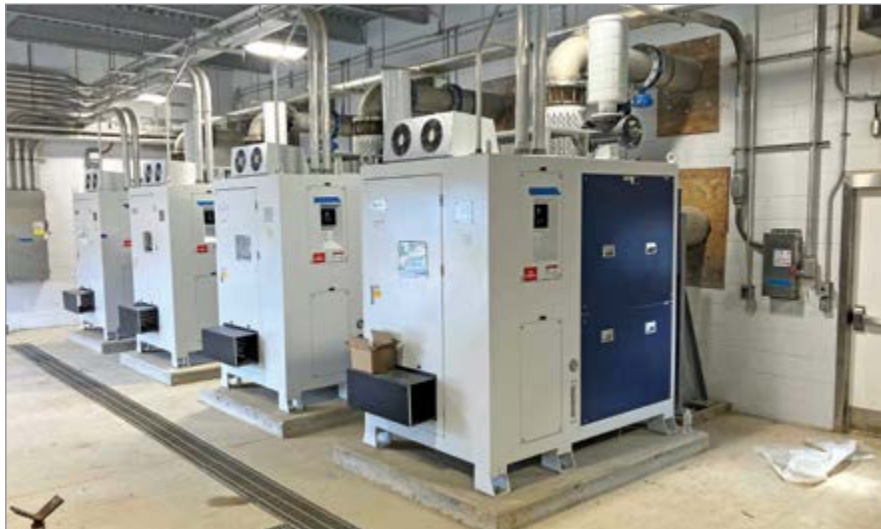
Four turbo aeration blowers at a major poultry producer.
