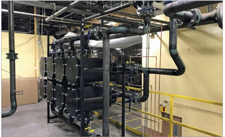
A centralized bank of particulate filters protecting a vacuum pump system.
