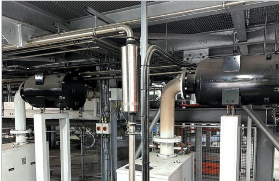
Point of use particulate filters protecting vacuum pumps.
