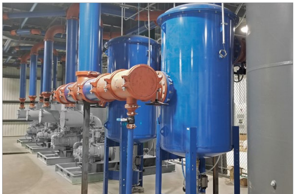
Two knockout tanks plumbed in parallel to protect a centralized bank of four vacuum pumps from ingesting liquids.
